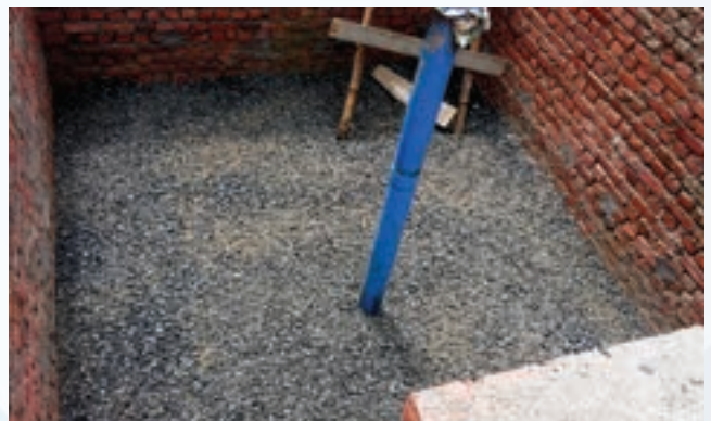
Roof water harvesting system to maintain ground water level
